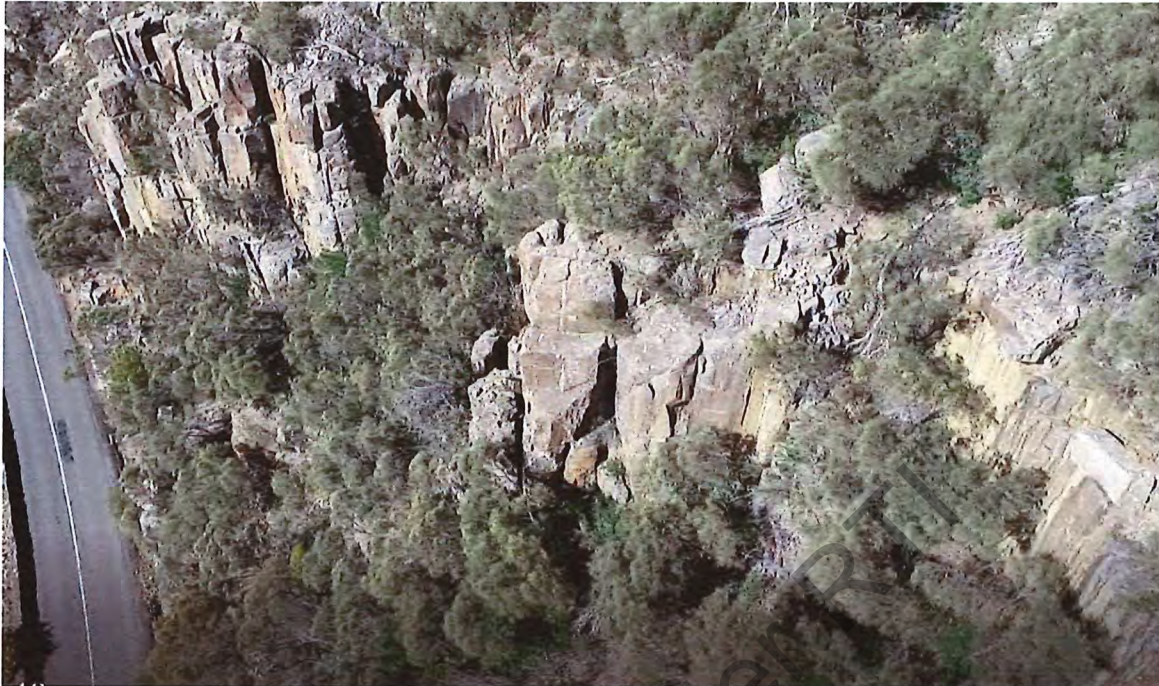
Figure 6: Buttress of interest back left; second buttress middle ground. More open cracking at top.
