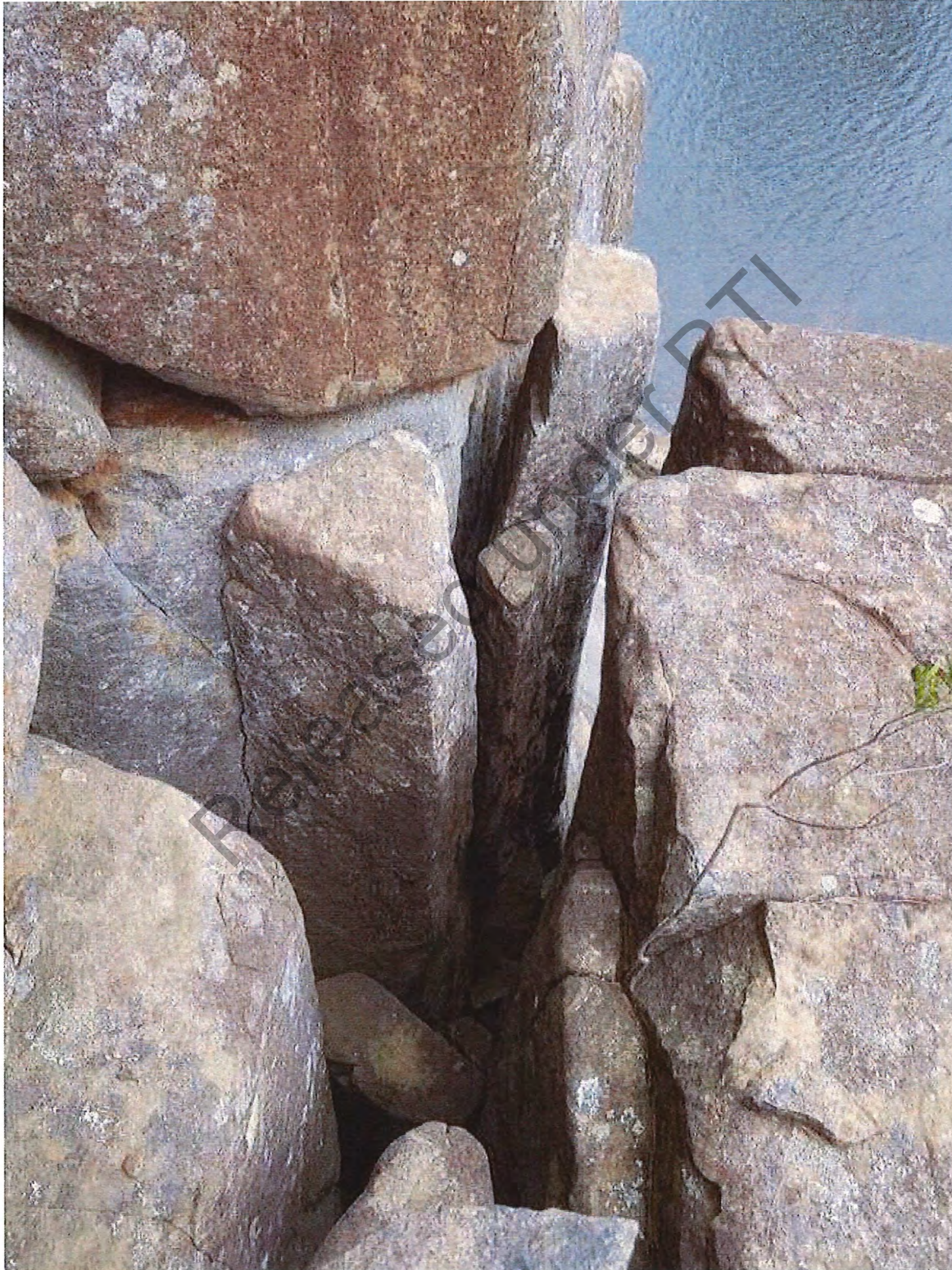
Figure 10: Open defects lower down buttress (restrained boulder is above boulder in upper left of photo)
