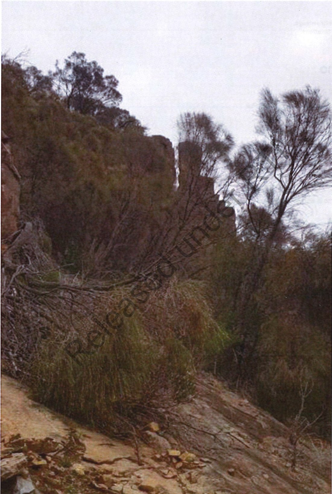
Figure 1: View of crack behind restrained boulder
