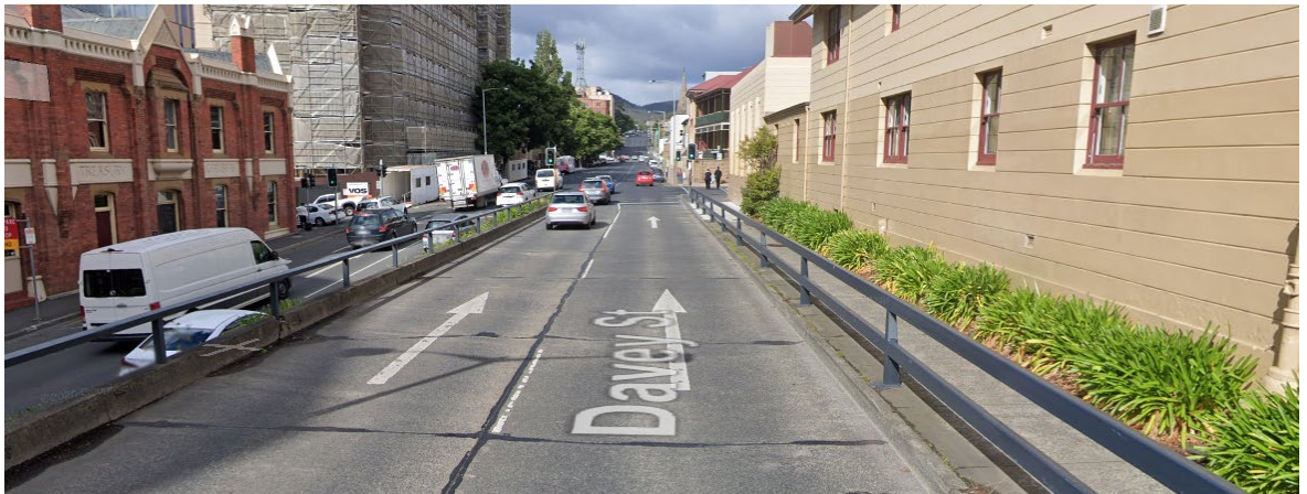
Figure 5 – Existing Barrier Type does not meet current standards
